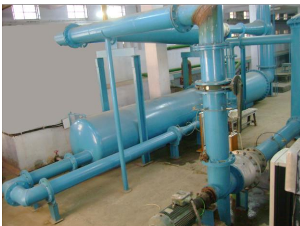
Fig 2. Pump Test Rig
